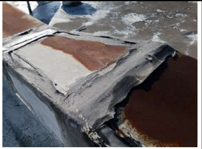
Photo 2: roof – mastic on HVAC ducts and penetrations (ACM)
