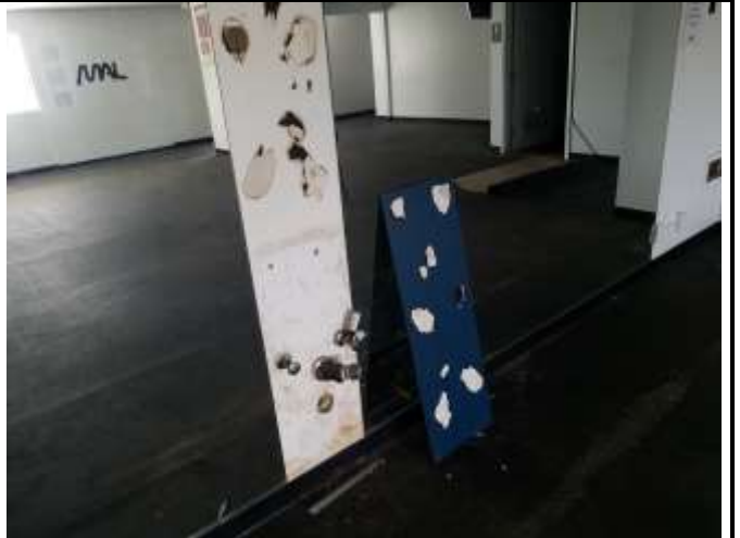
Photo 8: mirror mastic (ACM)
