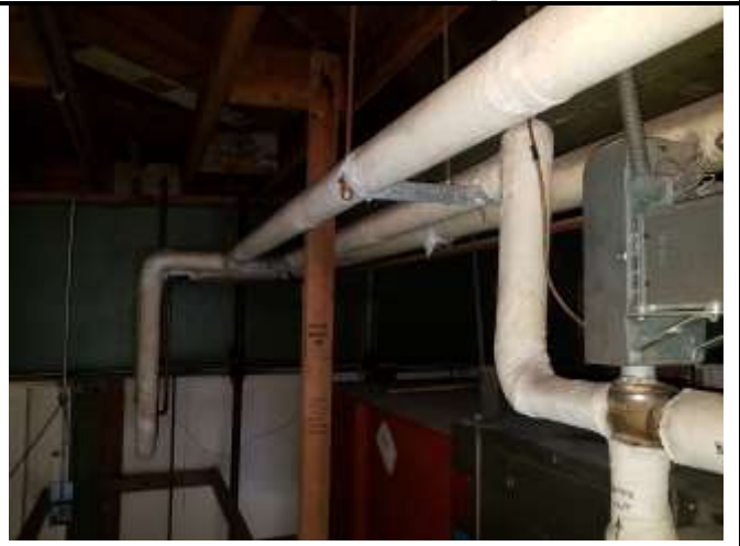
Photo 4: Attic/loft TSI pipe insulation (ACM)
